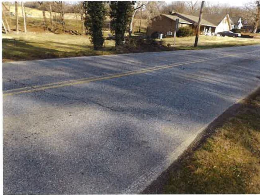
VIEW ACROSS DECK (NOTE: MINOR RAVELLING)
