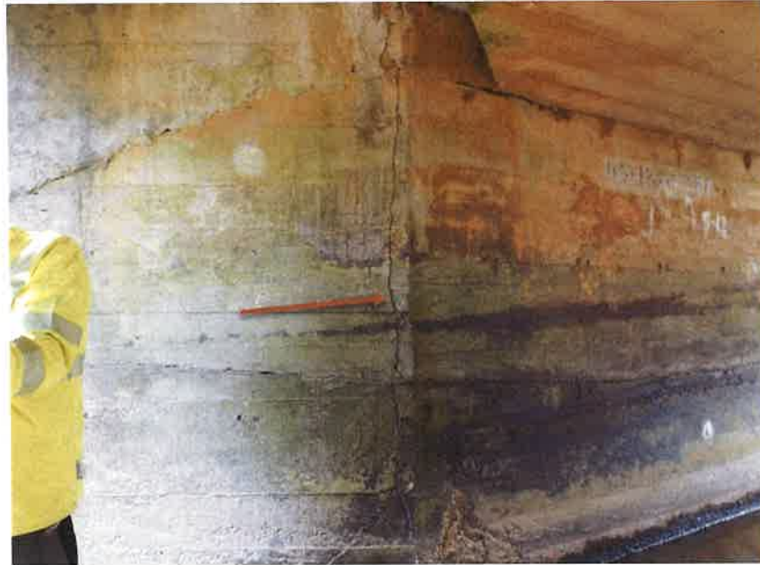
CRACK UP TO 1/8" OPEN WING 1 RIGHT
