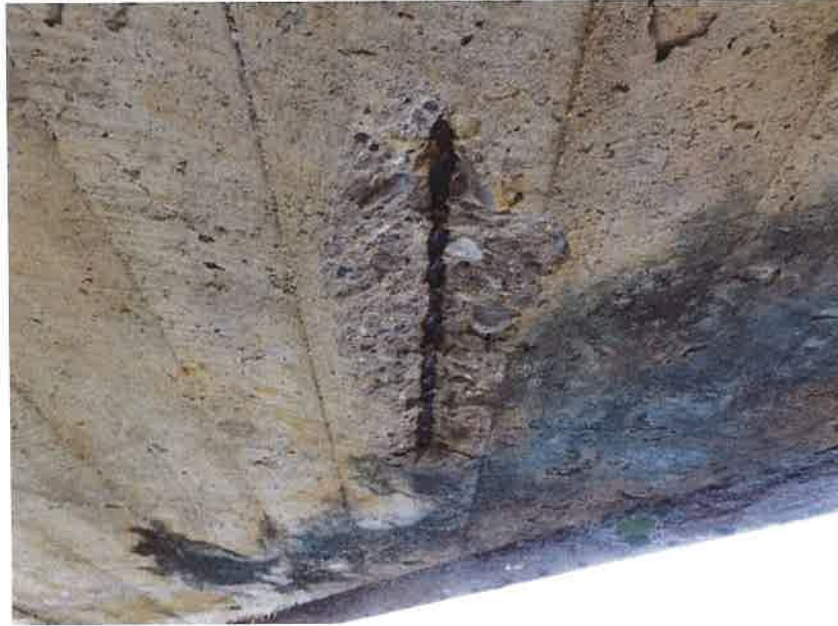
SPALL EXPOSED REBAR TOP BARREL 1 NEAR OUTLET
