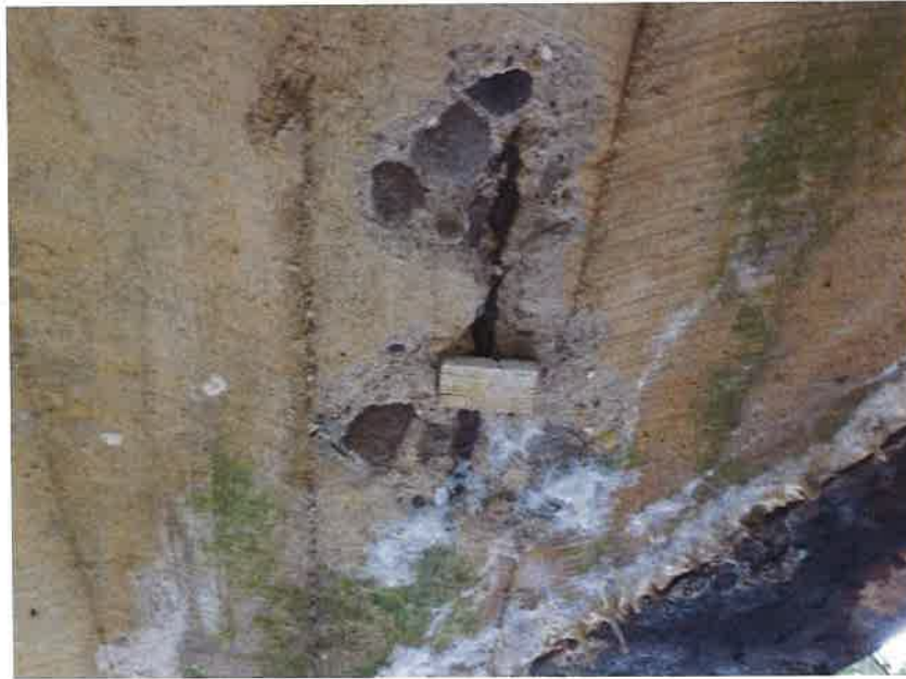
SPALL EXPOSED REBAR TOP BARREL 2 OUTLET
