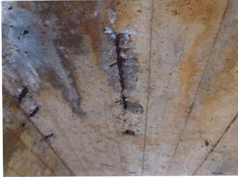
SPALLS EXPOSED REBAR TOP BARREL 2 NEAR OUTLET
