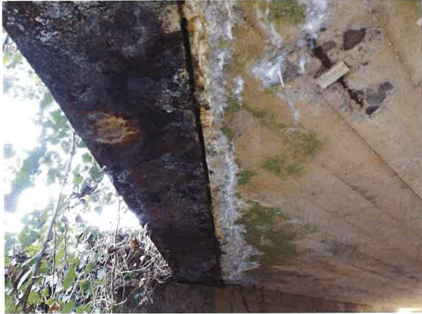
CRACK W/LEACHING TOP BARREL 2 OUTLET
