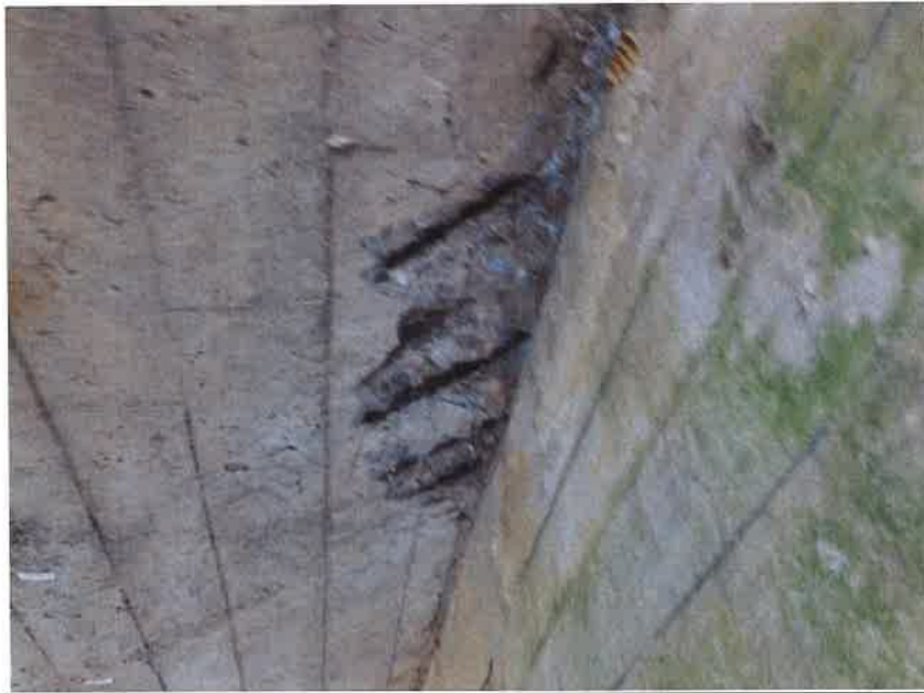
SPALL EXPOSED REBAR TOP BARREL 2 NEAR OUTLET
