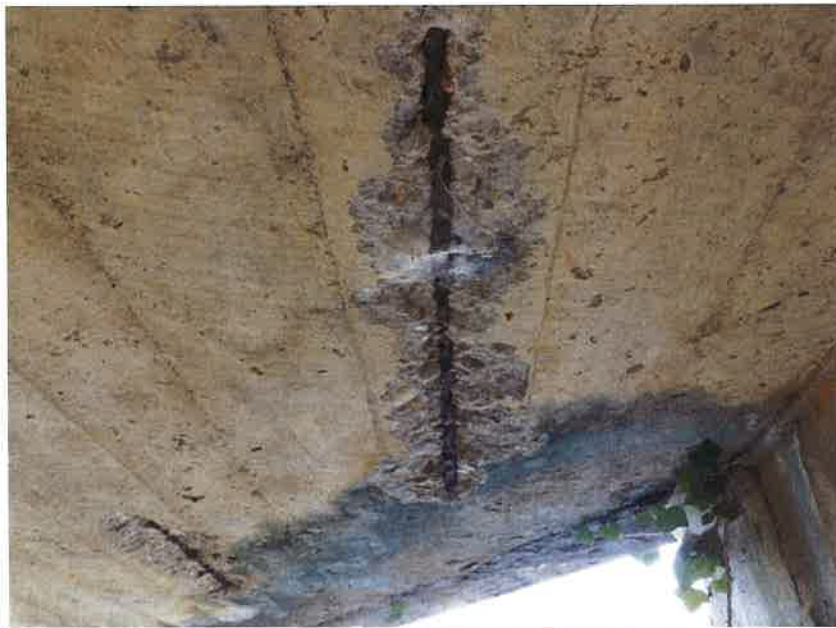
SPALLS EXPOSED REBAR TOP BARREL 1 NEAR OUTLET
