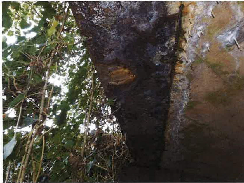
HEAVY CORROSION BEAM OUTLET
