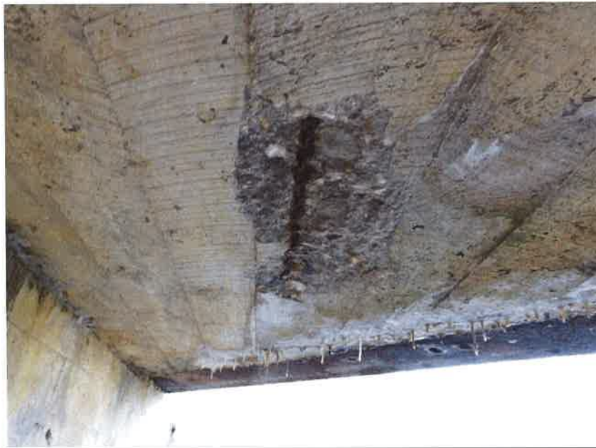
SPALL EXPOSED REBAR TOP BARREL 1 NEAR OUTLET
