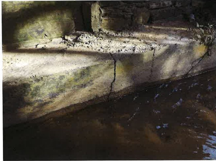
CRACK SILL ABUTMENT 2 NEAR INLET
