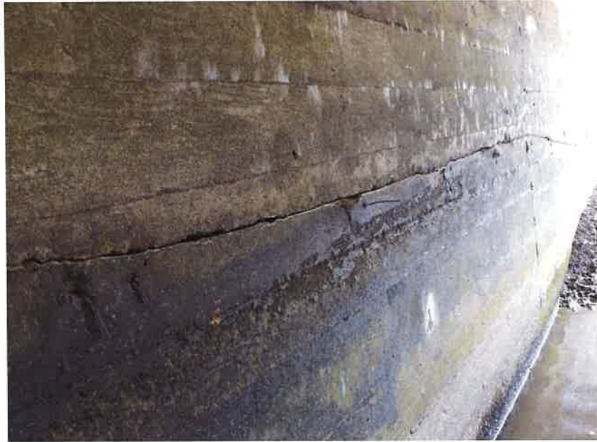
CRACK UP TO 1/8" OPEN BREASTWALL ABUTMENT 1
