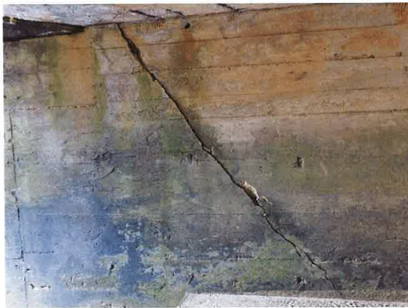
CRACK UP TO 1/2" OPEN BREASTWALL ABUTMENT 2
