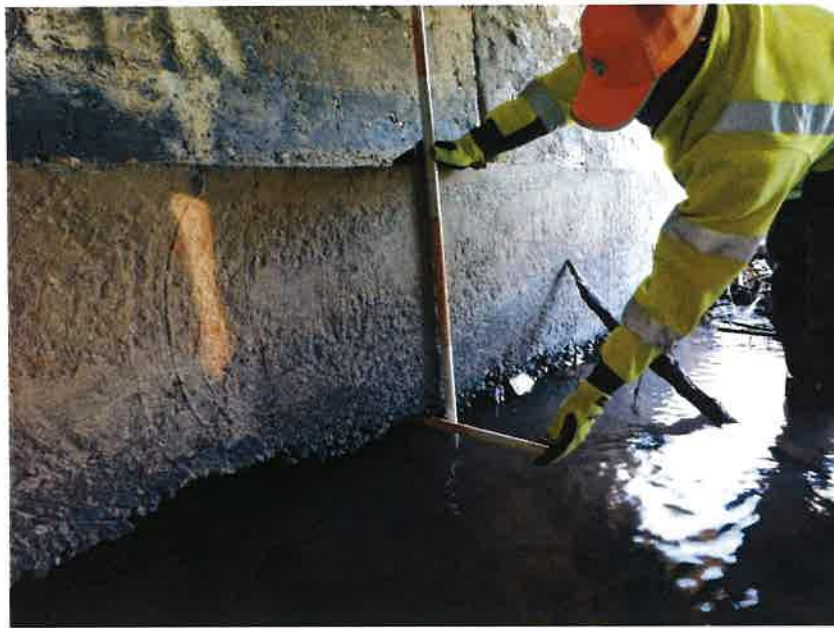
UNDERMINING UP TO 3' DEEP ABUTMENT 1 LEFT
