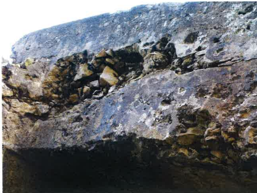
HEAVY SCALE HEADWALL OUTLET
