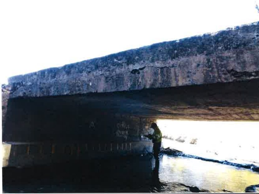
CRACK UP TO 1/4" OPEN HEADWALL OUTLET
