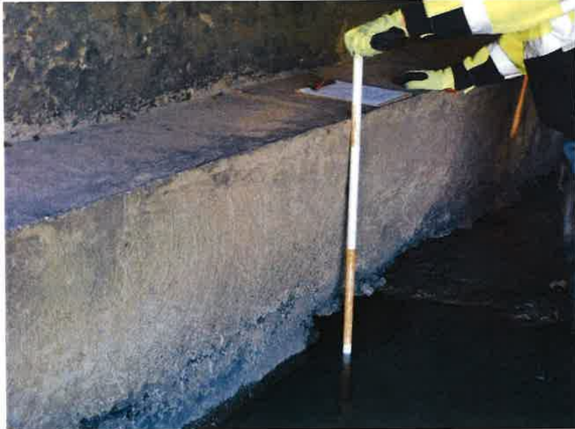
UNDERMINING UP TO 4' DEEP ABUTMENT 2 MIDDLE
