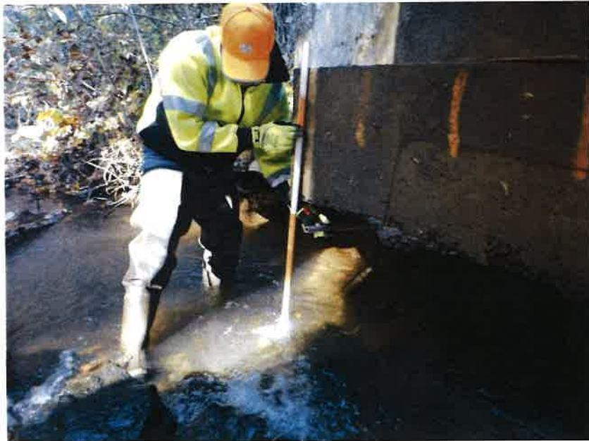
UNDERMINING UP TO 4' DEEP ABUTMENT 1 RIGHT
