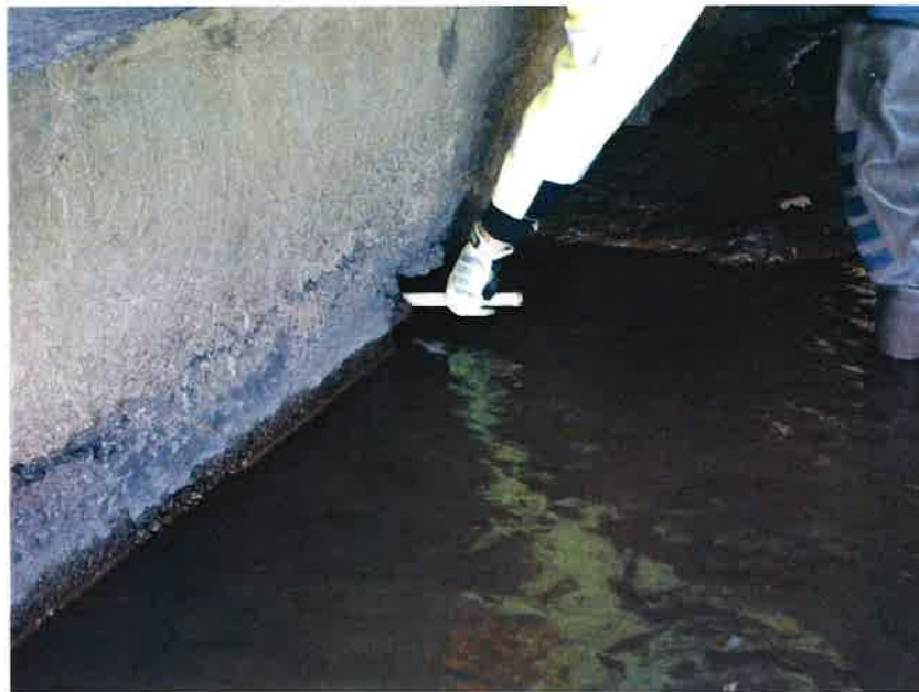
UNDERMINING UP TO 4' DEEP ABUTMENT 2 MIDDLE
