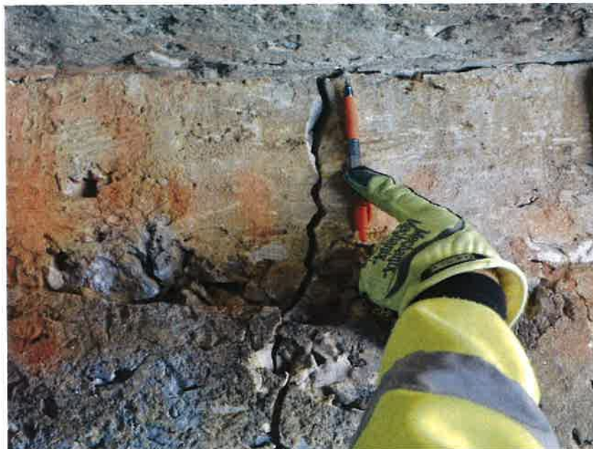
CRACK UP TO 3/8" OPEN BREASTWALL ABUTMENT 1
