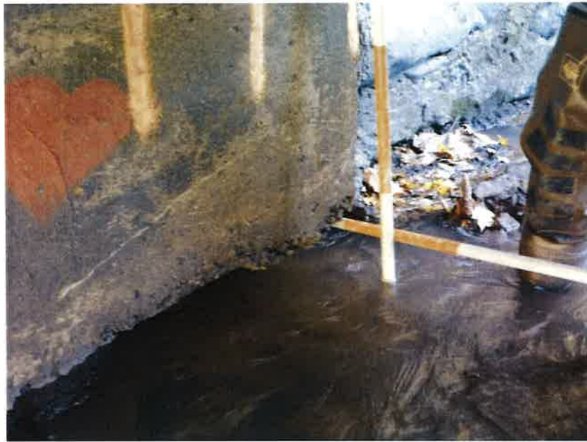
UNDERMINING UP TO 1' DEEP ABUTMENT 2 LEFT
