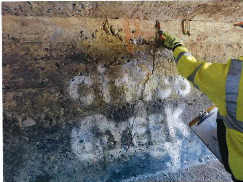
CRACK UP TO 3/8" OPEN BREASTWALL ABUTMENT 1
