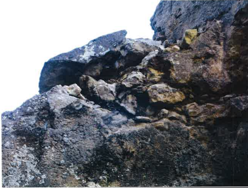
SPALL 1' DIAMETER 4" DEEP TOP WING 1 RIGHT
