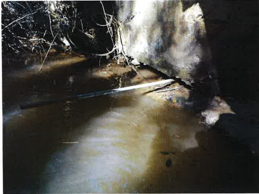
UNDERMINING AT WING 1 RIGHT OUTLET
