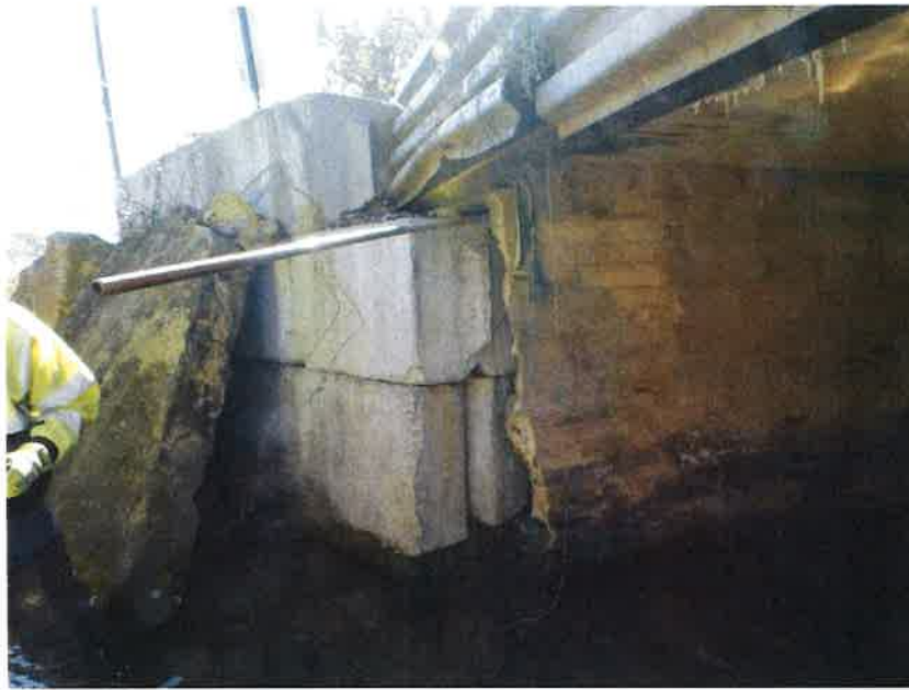
VOID BEHIND WING 2 LEFT
