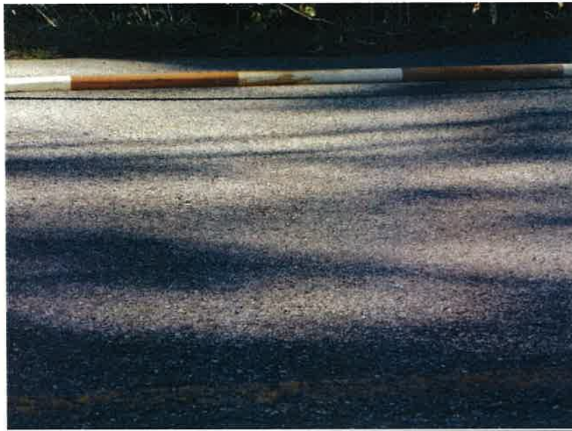
SLUMPING/SETTLEMENT AT APPROACH 1 RIGHT
