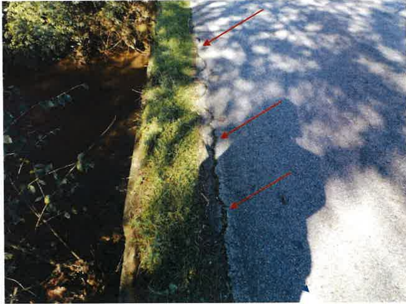
ROTATION OF RIGHT HEADWALL NOTE SEPARATION CRACK
