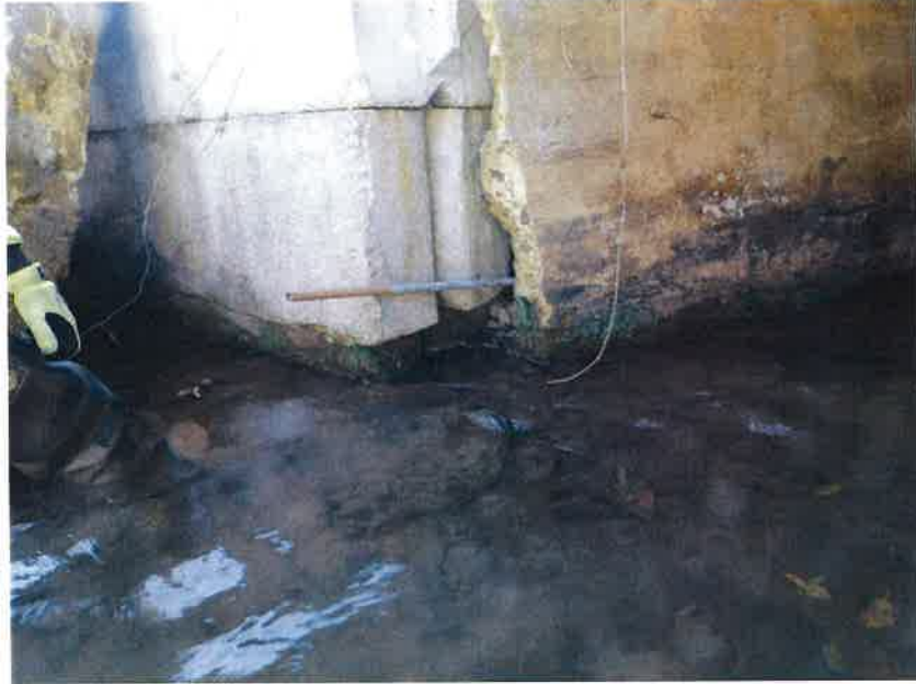
VOID BEHIND ABUTMENT 2 AND WING 2 RIGHT
