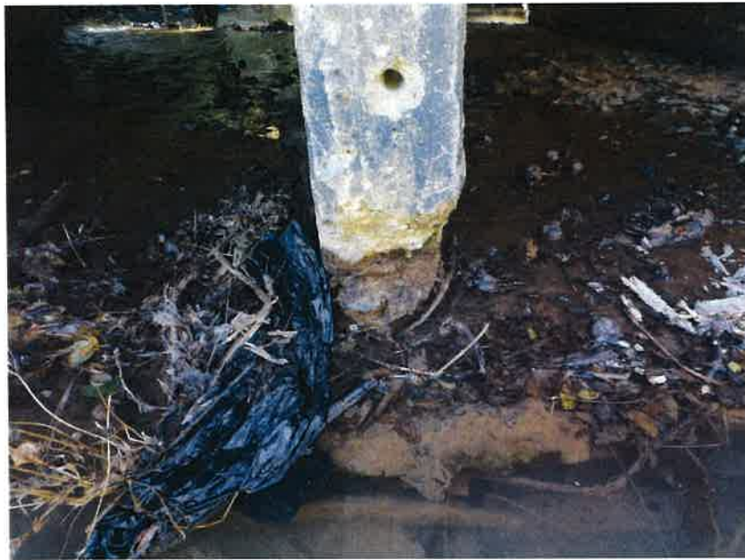
SCALE AT MIDWALL INLET WATERLINE
