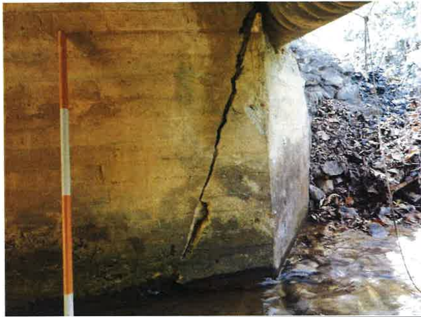
CRACK AND ROTATION OF WING 2 RIGHT
