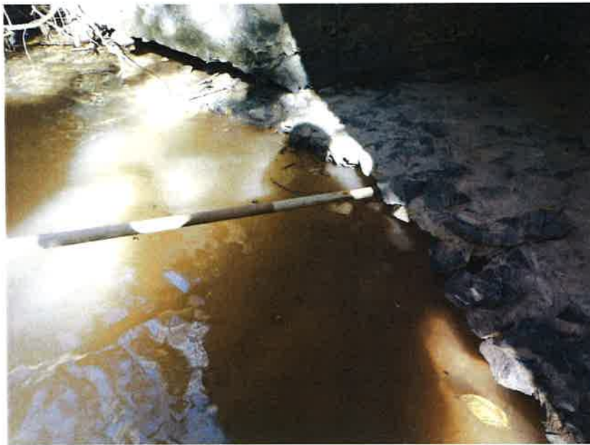
UNDERMINING AT BARREL 1 OUTLET
