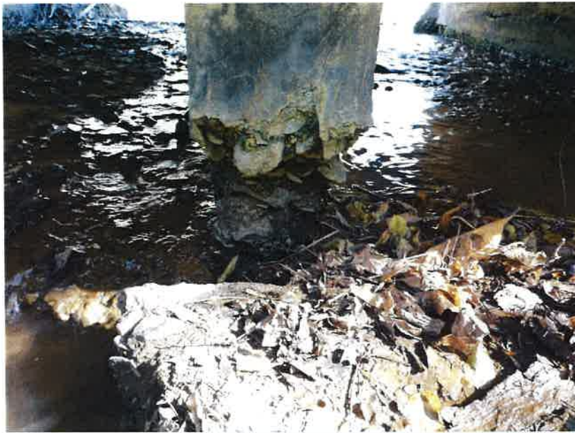
HEAVY SCALE MIDWALL AT OUTLET WATERLINE
