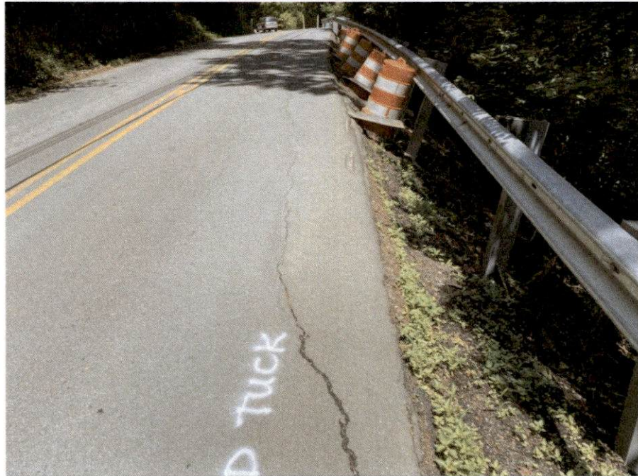
Figure 2 – Conditions along Old Tuckaleechee Road in August 2022
