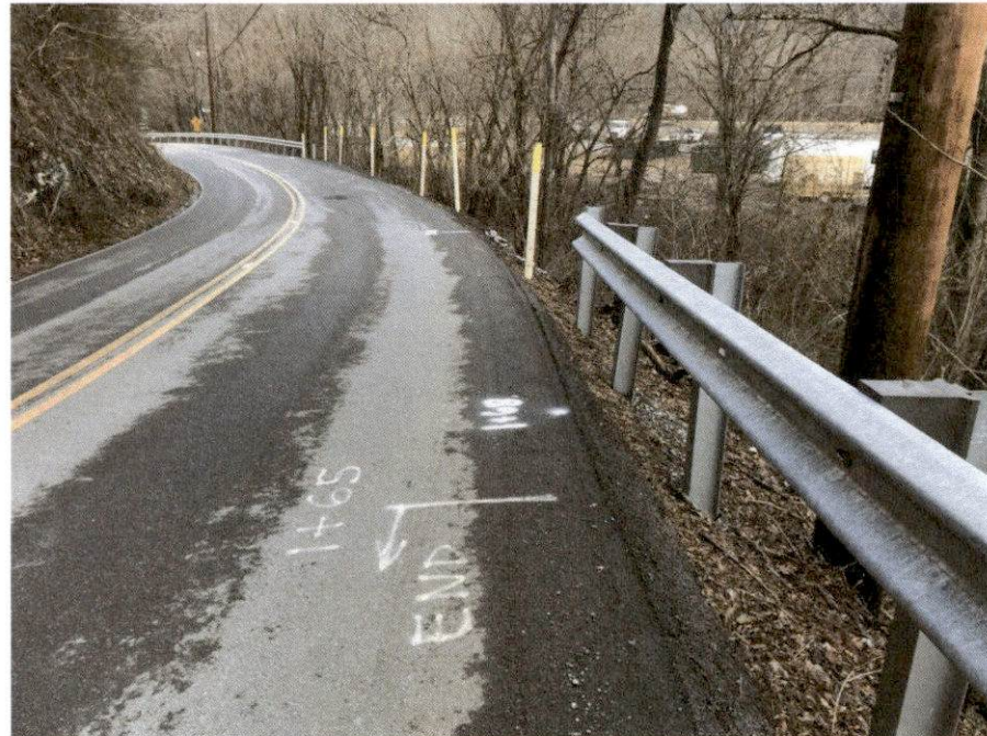
Figure 3 – Existing conditions along Old Tuckaleechee Road as of January 2023, past the end of the August 2022 repair
